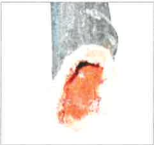
Corrosion build-up in metal pipes
